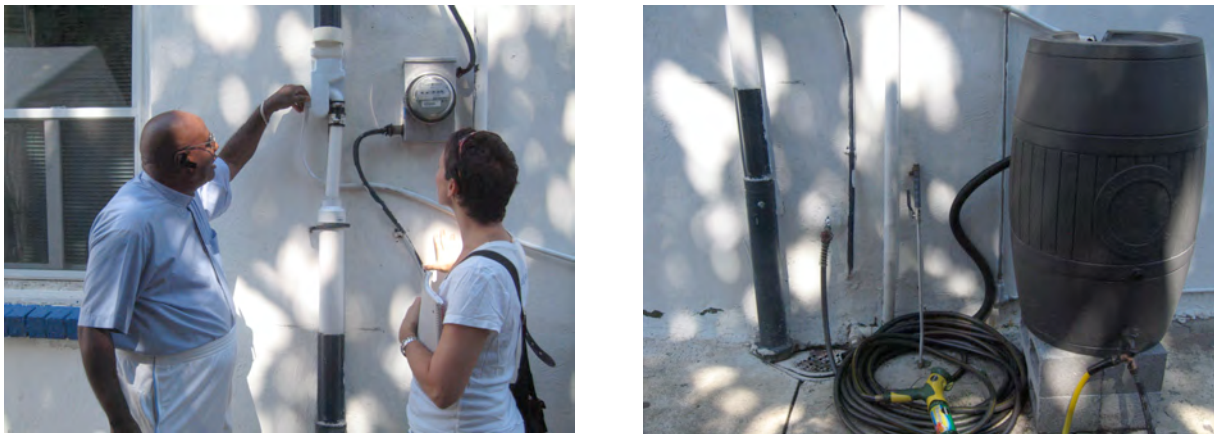
Figure 5 – Rain barrel installation at a Philadelphia home
